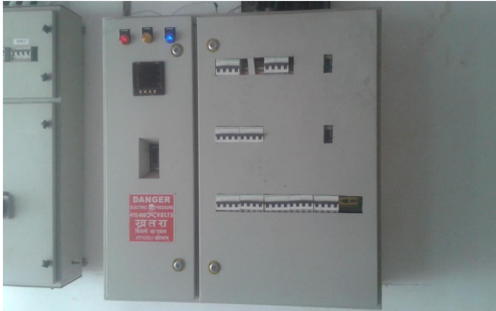
Incoming feeder of solar
