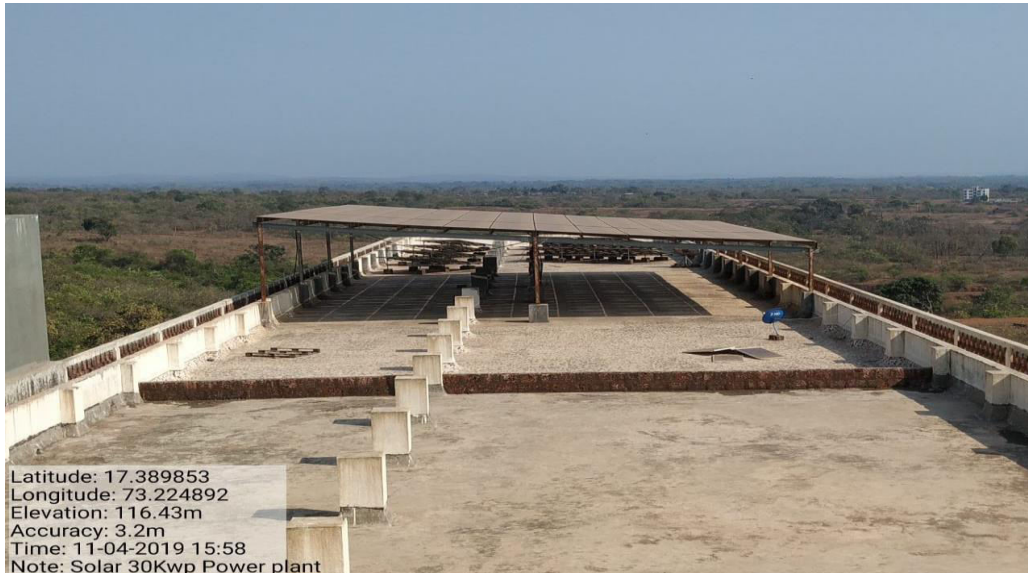
30Kwp Solar on Sripati A1 Building
